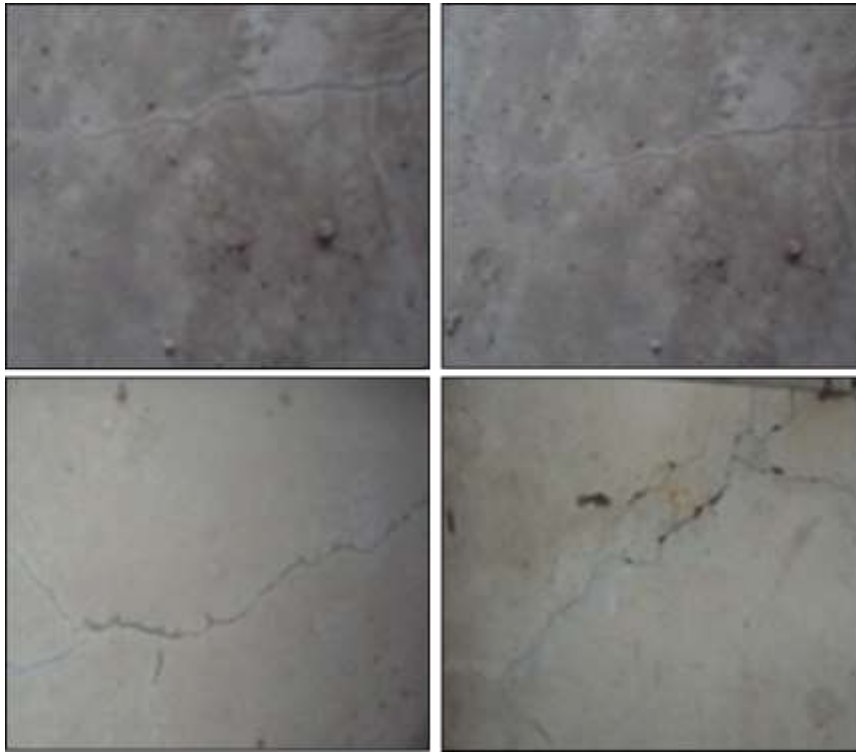
Figure 2. Damages in the constructed structures due to the heaving of soil.
